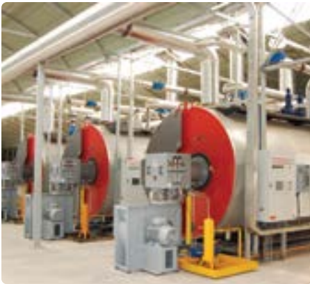
Hot Water Heating
